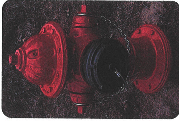
All Hydrants are Inspected & Tagged
