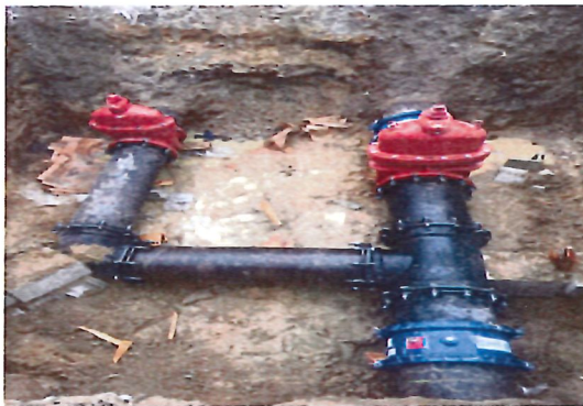
New Valves on a 12" & 16" Main Distribution Line
